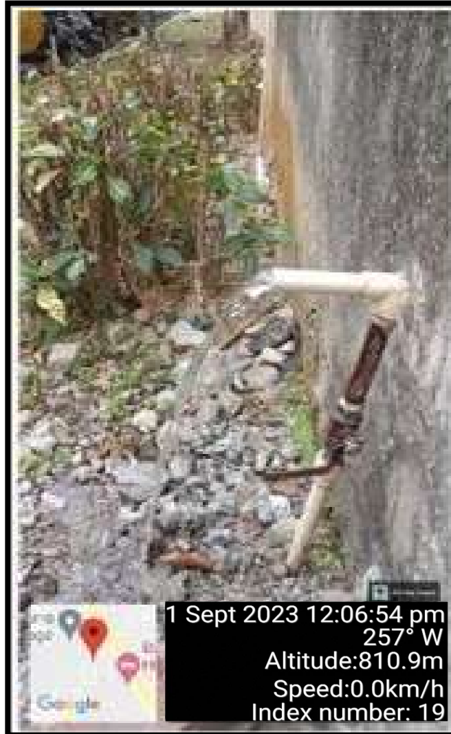
Figure 4-28: STP treated water tap for garden use
